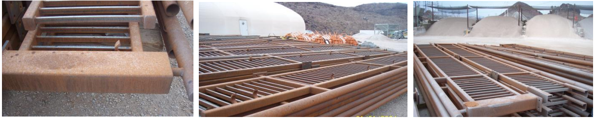
Steel railings were allowed to develop flash rust in preparation for the Rust Grip® application.
