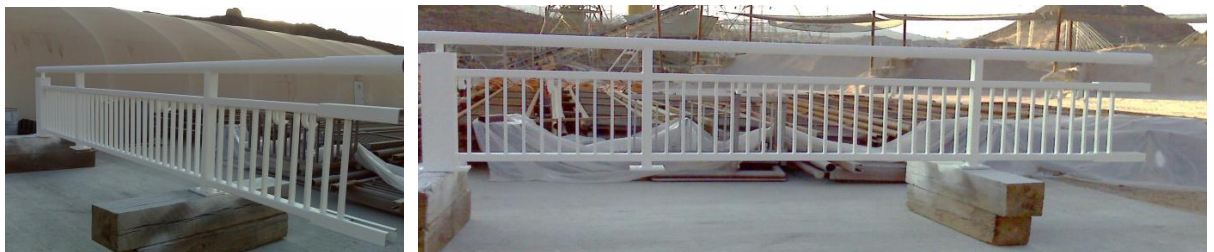
Super Therm® was applied to prevent heat from loading onto the steel railings, possibly burning visitors.
